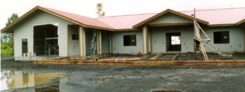
The west-facing façade with the main entry in center and the workshop on the left.
